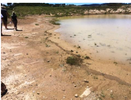
Tide lines suggest dam leakage
